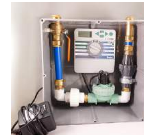
Irrigation Control Unit w/ fertilizer injector system
